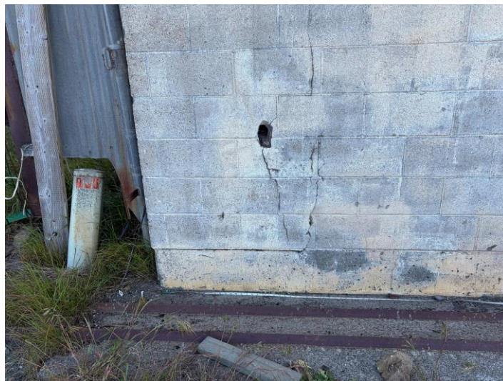
Figure 10: Boat Yard – Cracked CMU wall.
