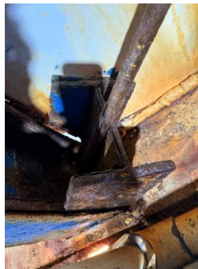
Figure 22: Fish Processing Facility 1 – Corroding Lateral Bracing.
