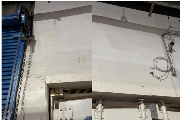
Figure 25: Fish Processing Facility 1 – Cracking finished material above shipping containers cut into the north exterior wall.
