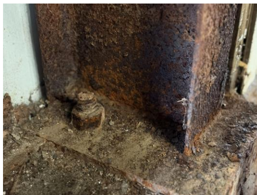
Figure 52: Storage Building – Failing column post.
