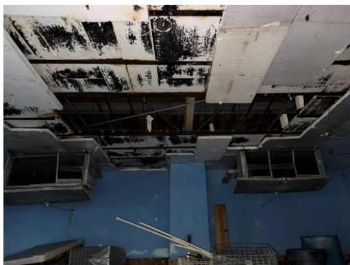
Figure 30: Fish Processing Facility 2 – Degrading mechanical refrigeration units, and refrigeration insulation.
