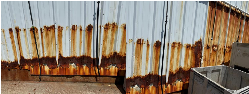
Figure 18: Fish Processing Facility 1 – Deteriorating exterior siding causing framing members to fail.
