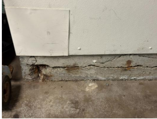
Figure 26: Fish Processing Facility 1 – Cracking concrete curb, with rust stains coming from the cracks.
