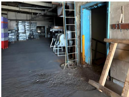
Figure 29: Fish Processing Facility – Degraded concrete slab and curb.
