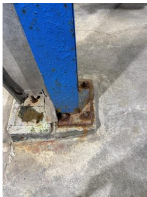
Figure 19: Fish Processing Facility 1 – Interior column base with corroding base plate, and bubbling paint.
