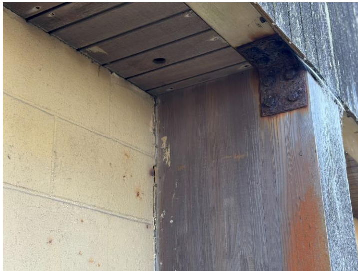
Figure 6: Boat Yard – Corroded Hardware on north side of the structure.
