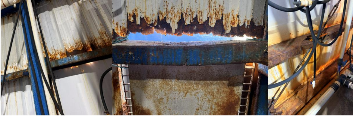
Figure 17: Fish Processing Facility 1 – Extreme deterioration in wall girts along south-west corner.
