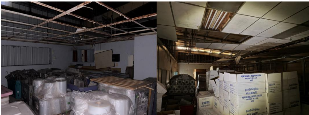
Figure 28: Fish Processing Facility 2 – Degrading drop down ceiling.
