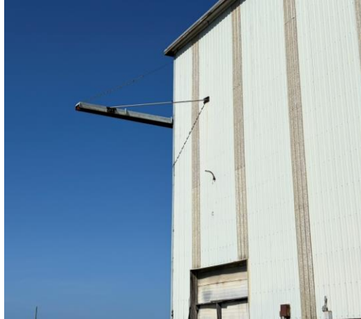
Figure 12: Boat Yard – Access Door Frame
