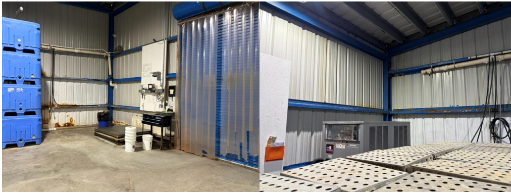
Figure 23: Fish Processing Facility 1 – Missing or not visible bracing from secondary edition.
