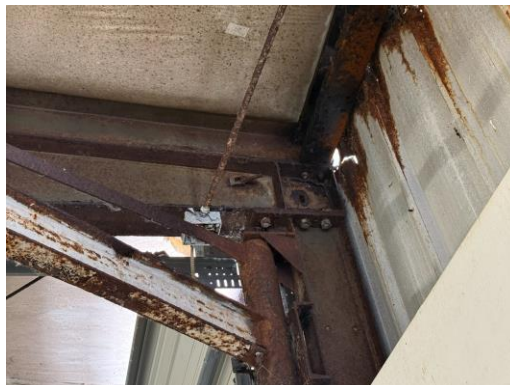
Figure 48: Storage Building – Rusting roof eave members.
