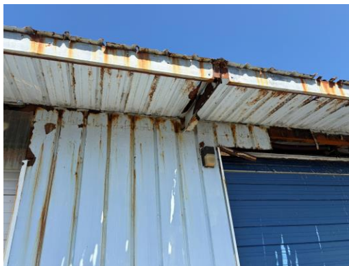
Figure 49: Storage Building – Rusty exterior siding.
