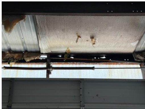
Figure 51: Storage Building – Degraded exterior doorway framing.
