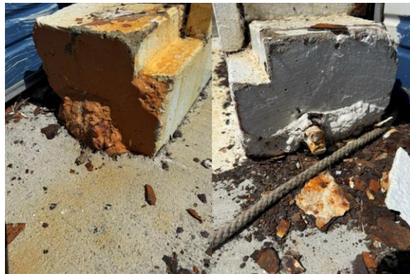
Figure 53: Storage Building – Cut concrete curb, and corroding reinforcement.
