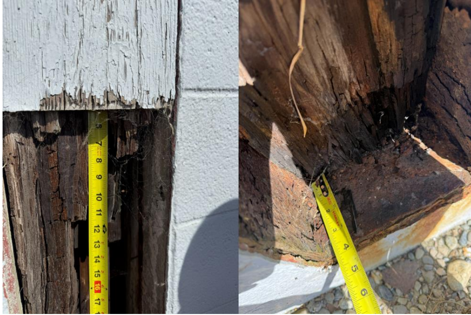
Figure 5: Boat Yard – Damage to exterior wood post along south side of the structure.
