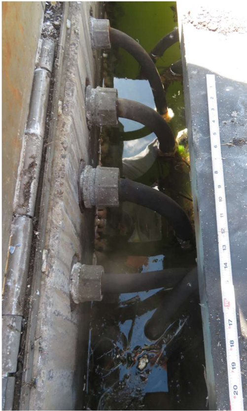
a) Wiring at HM01 to 02
