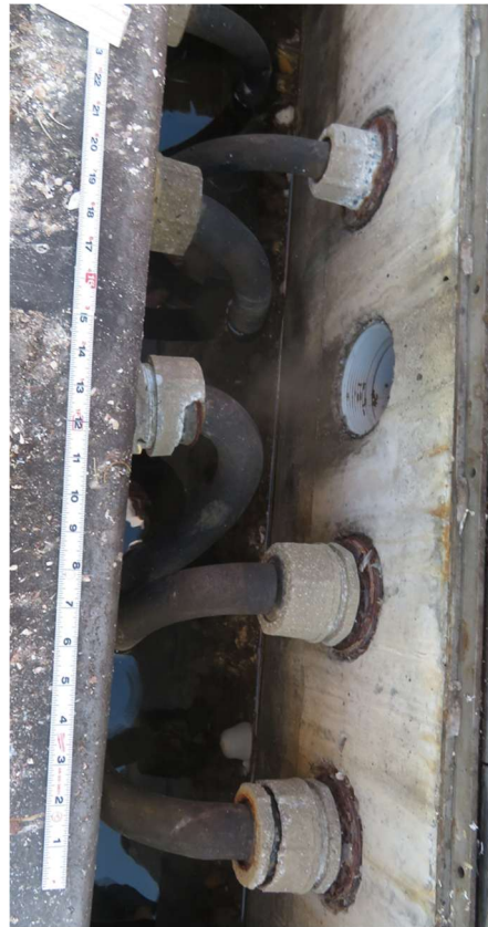
b) Wiring at HM03 to 04
