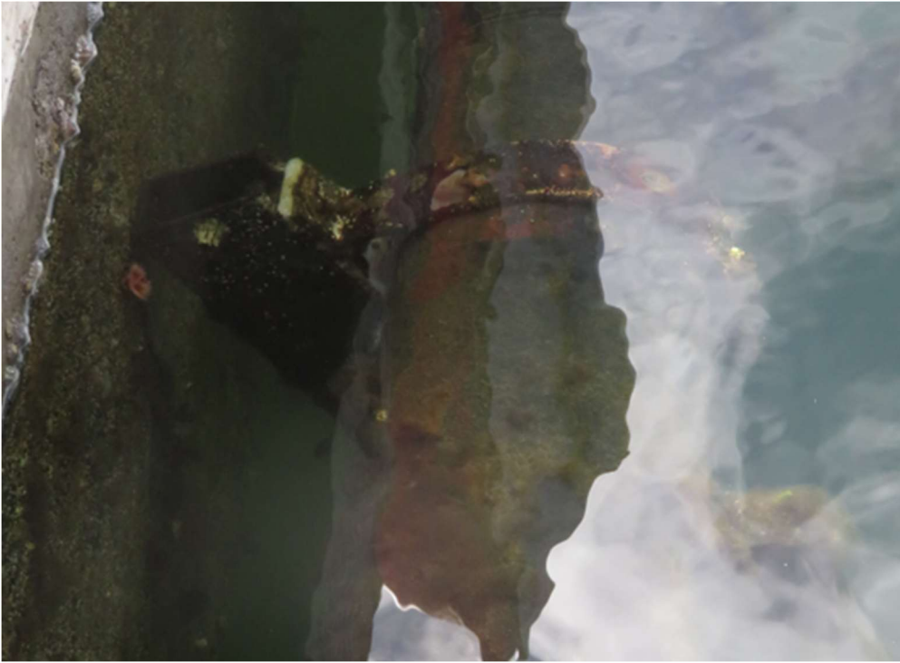
Figure 7: Example Loss of Firewater Pipe Support (Not at Dock H)
