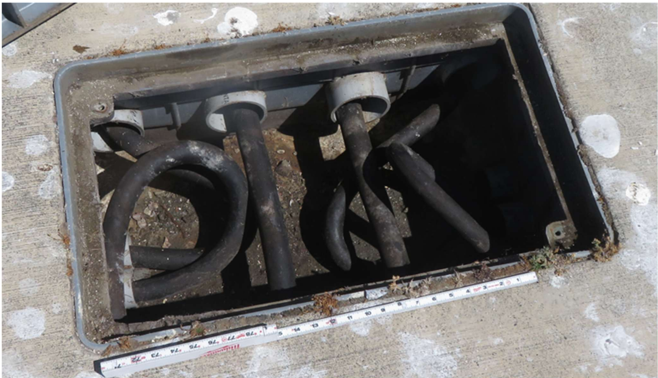
Figure 5: Wiring at Pull Box on HM01
