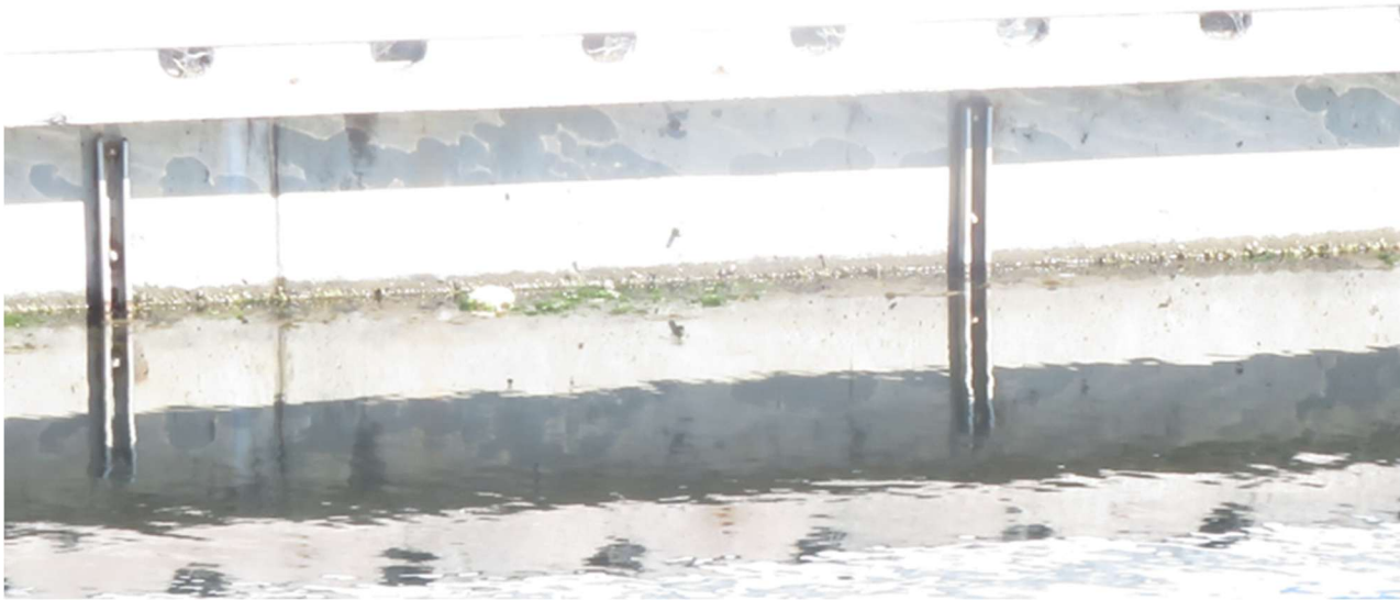
Figure 16: Example of retrofit Unistrut above the waterline
