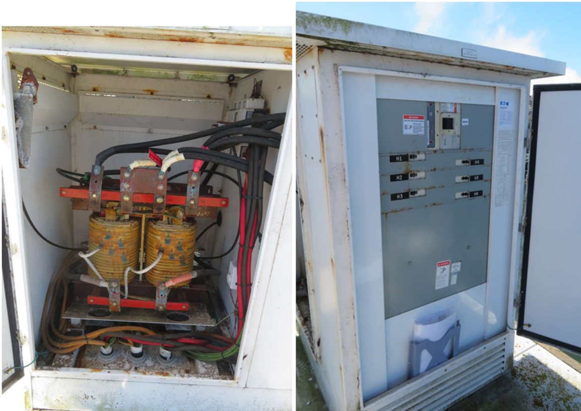
Figure 4: Combined Transformer and Load Panel at float MM08
